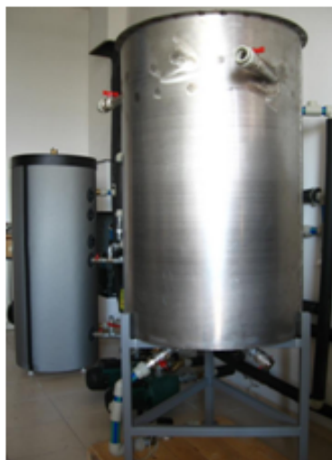
Figure 2 – Latent heat storage which contains 39 PCM containers filled with E53
